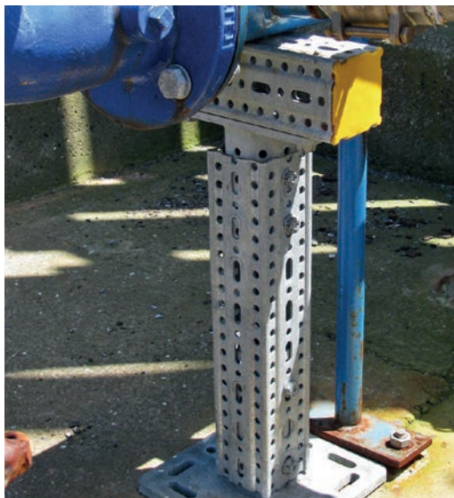
Conventional and siFramo 80 T-supports A few months after installation
